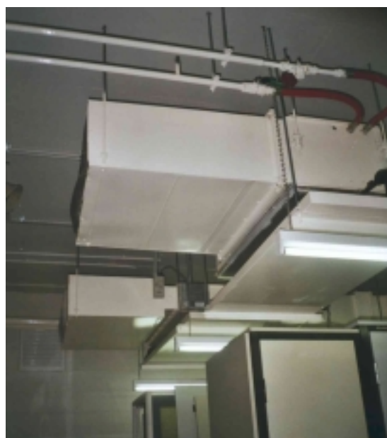
Air-conditioning units in ER area
