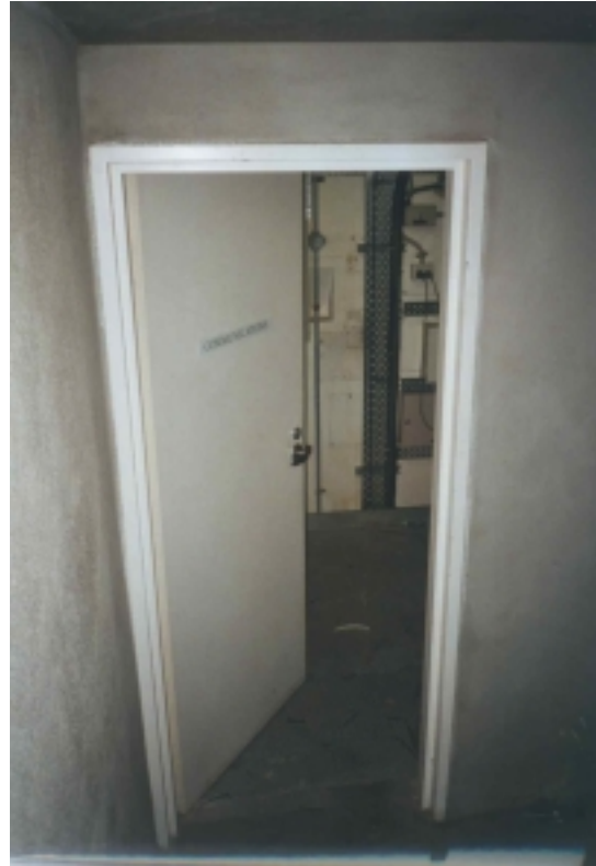
Sufficient access should be provided into riser shafts
