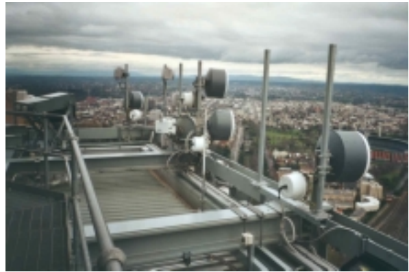
Radio Communications on rooftop
