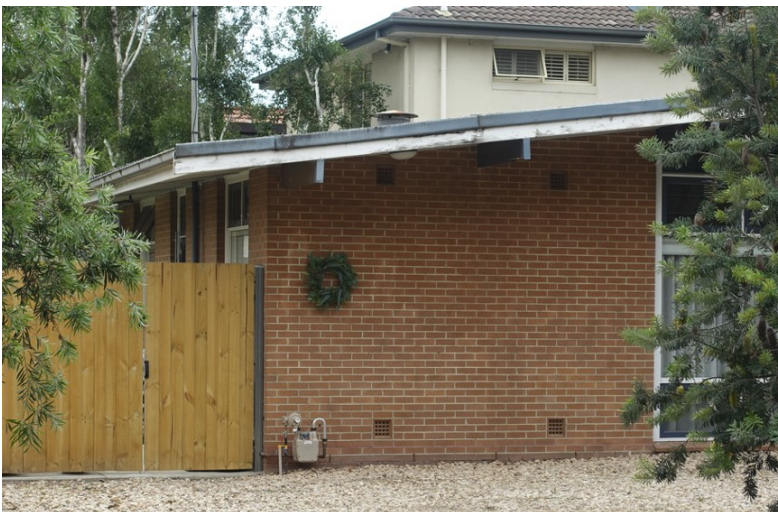
Figure 5. Brickwork to part of the front elevation and the east side elevation, Dec. 2023. (N Schmeder)
